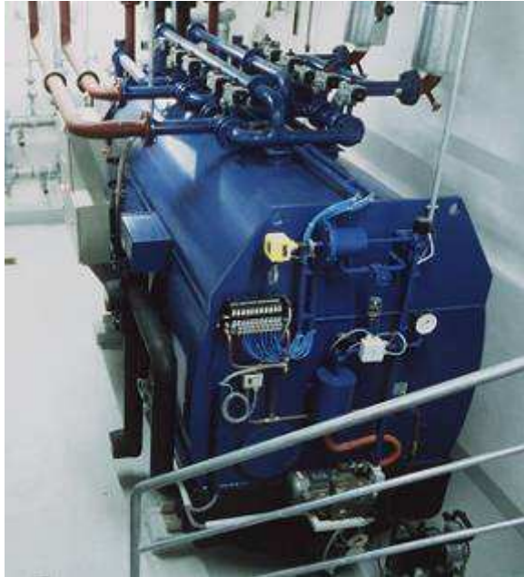
Nishiyodo NAK 70 kW chilling capacity Installation: University hospital Freiburg, Germany
